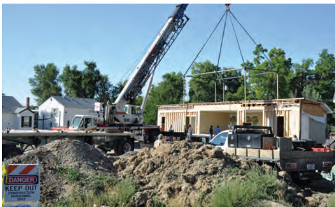
Billings, Yellowstone County • Rimrock Foundation $610,000 in bonds to refinance three existing loans, install a chiller system and build a basement for a new modular facility. Benefit: Reduce interest expense and expand services to better serve the underserved population in Montana.
